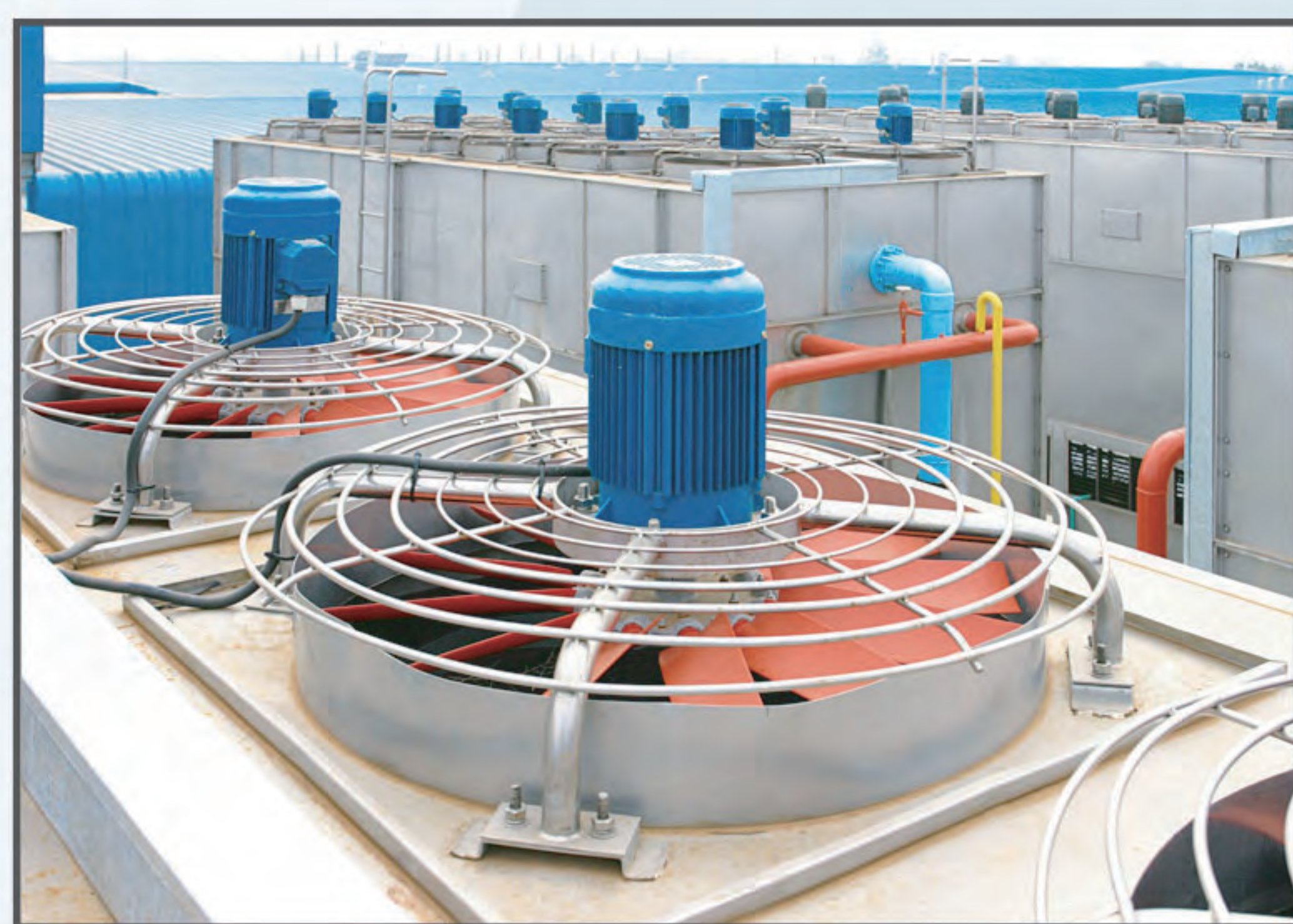
Fan and water pump
